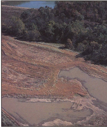
The area where dirt was taken for the dam will be an extensive wetland.
